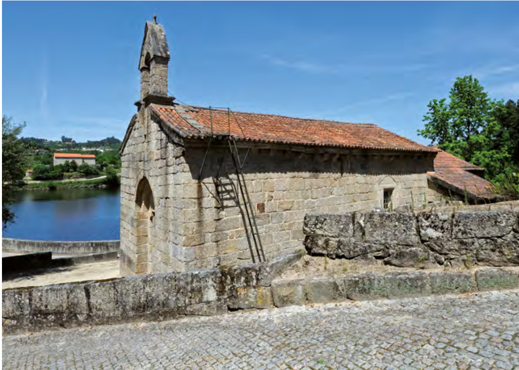
Church of Saint Nicholas (Marco de Canaveses). West and south façades. On the background, the Church of Sobretâmega (Marco de Canaveses).
