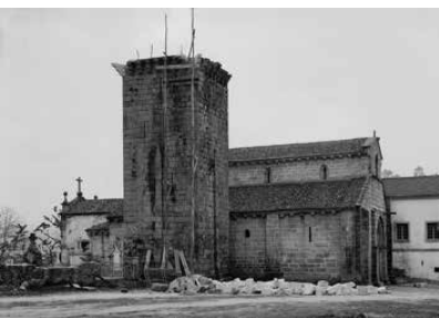
Church and tower during the intervention carried out by the DGEMN. Source: IHRU archive.
