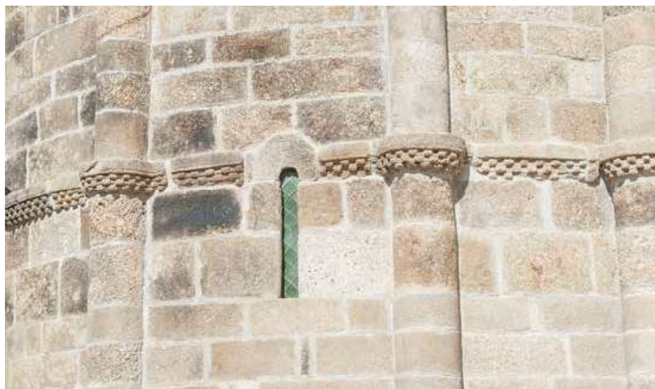
Church. South apse chapel. Frieze and crevice.
