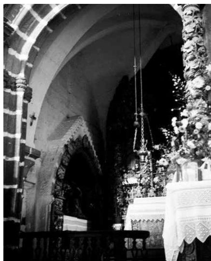
Church. Chancel. Arch connecting the chancel to the sacristy before the intervention carried out by the DGEMN. Source: IHRU archive.
