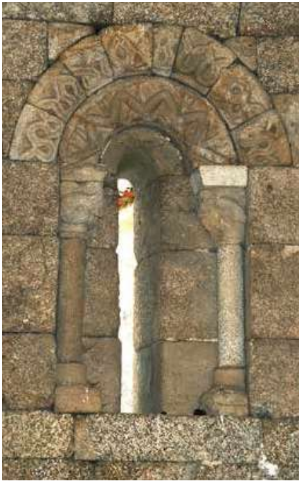
Pantheon of the Resendes. East façade. Interior view of the crevice.
