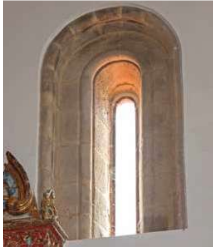
Church. South façade. Nave. Crevice. Interior view.
