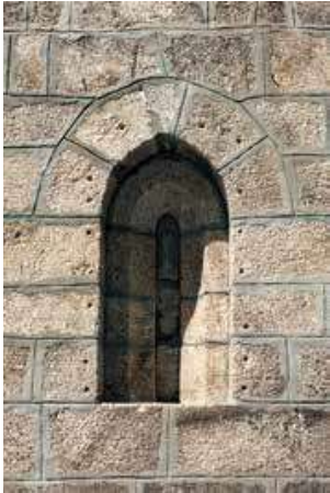
East façade. Crevice.
