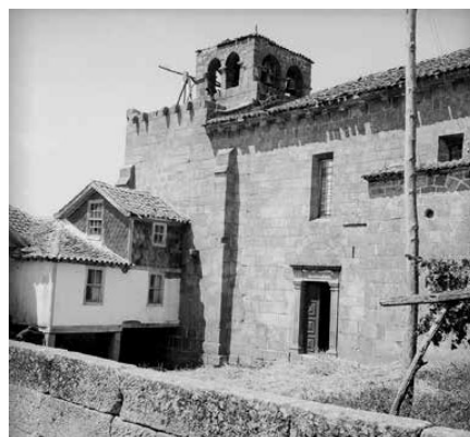
South façade before the intervention carried out by the DGEMN. Source: IHRU archive.
