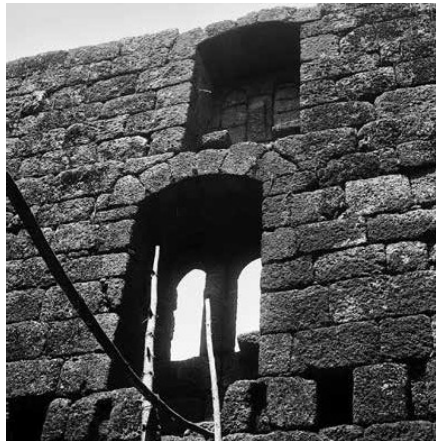
Northeast façade. Intermediate floor. Detail of the mullioned window (interior view) (1951). Source: IHRU archive.
