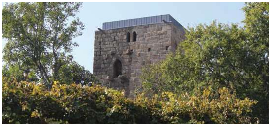
Northeast façade during the intervention carried out by the Route of the Romanesque (2014).
