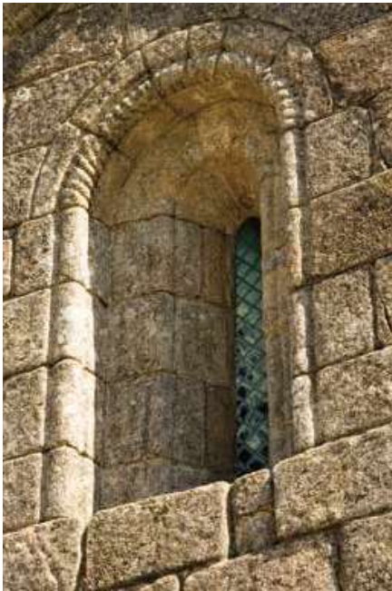
Church of Cabeça Santa (Penafiel). West façade. Crevice.
