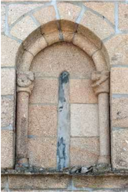
East façade. Crevice.
