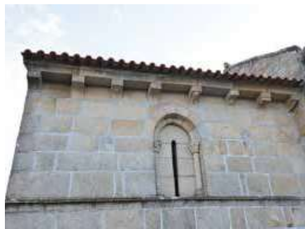
North façade. Corbels and crevice.
