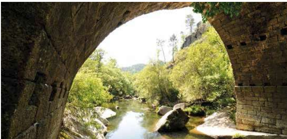
Detail of the constructive mismatch.
