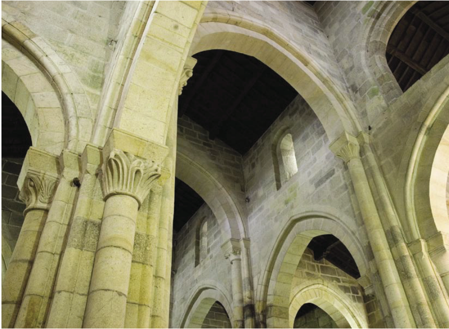
11. Transept roofing of the central and lateral naves. The diaphragm arches alternate with wood cover.
