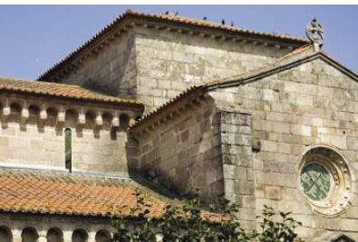
14. The transept's upper portion and the tower over the cross correspond to the last construction stage.
