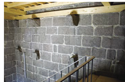
5. Projecting corbels subsist inside the Tower. They used to be the supports for the four stories high roofing framework.
