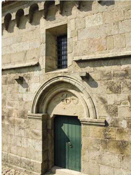
7. South façade. The drip course and corbels testify to the presence of a one story high porch or a cloister.
