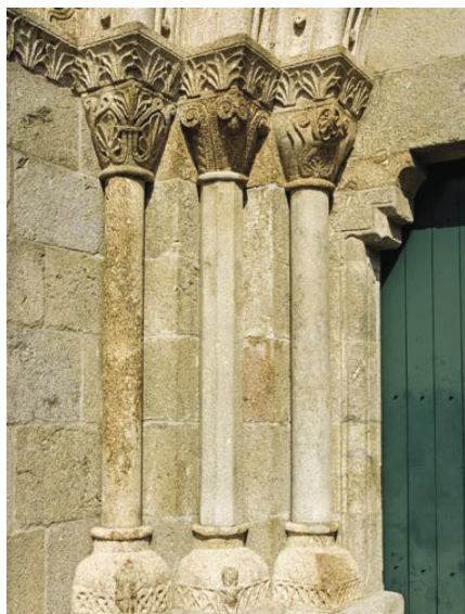
2. West portal. The capitals and the lines of ashlar, featuring vegetal themes, are examples of a current forged in the Sousa Valley, based in the Pre-Romanesque tradition and influenced by themes from Coimbra and of the See of Porto.
